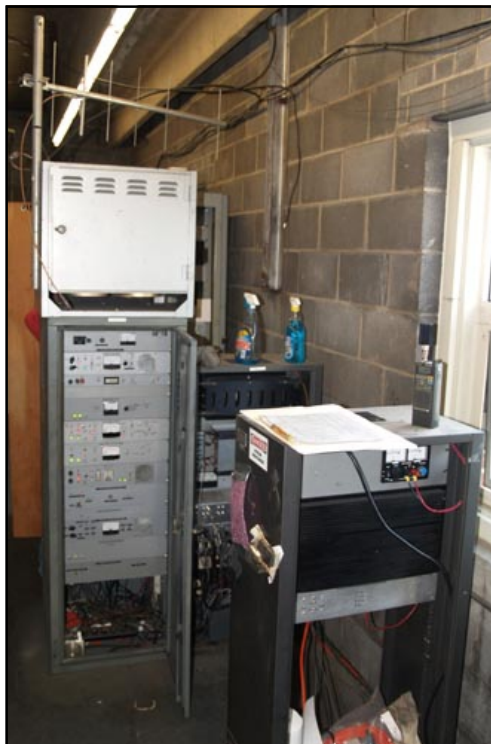
Above: Overview of the site. Backup transmitter cabinet is in foreground, main repeater rack on the left with duplexer cabinet on top; main transmitter cabinet is to the right, behind the backup transmitter. Control cabinet is behind the main rack.
