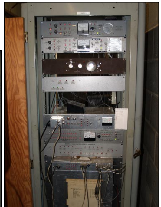
Above: Control cabinet. Contains receiver voter, link receiver, weather receiver, and control systems. Backup battery bank is in the bottom of this rack. More pix on Page 5!
