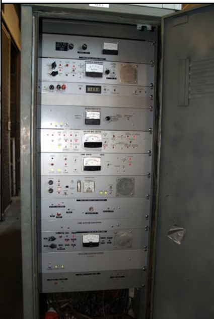
Below: Main repeater rack. Contains the #1 receiver, transmitter exciter and intermediate power amp, control receiver and some other neat gadgets.
