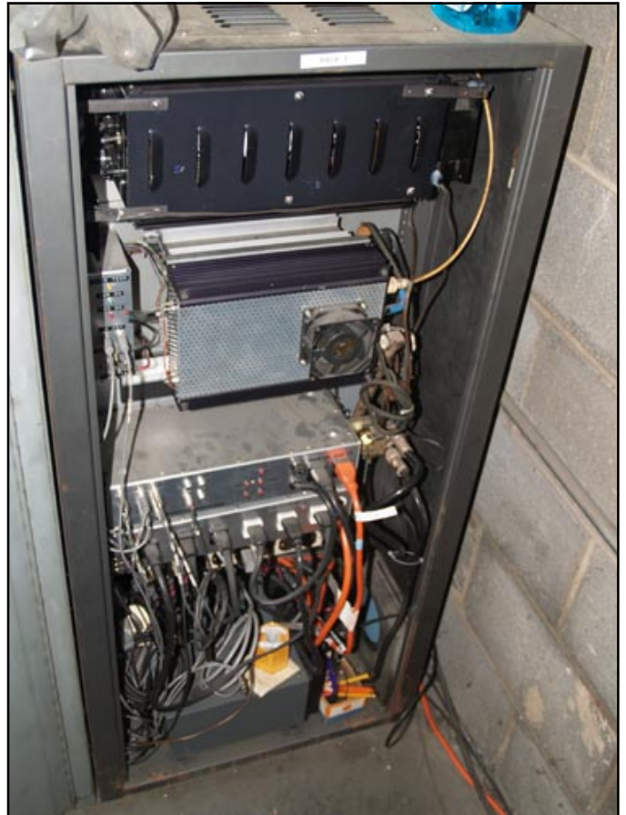
Above: Main transmitter amplifier rack. Power supply (top), amplifier (middle) and antenna and backup transmitter switching equipment (bottom).
