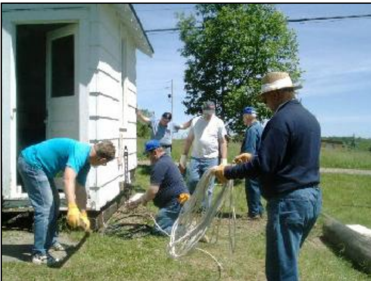
Getting ready to set the east side of the shack down on the tie.
