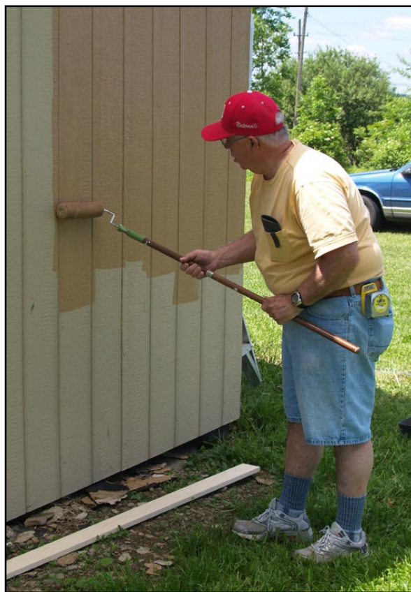
June 2007 found Bruce, WA2HVE, applying paint to the newly installed siding on Chet's Shack at Cole Road.
